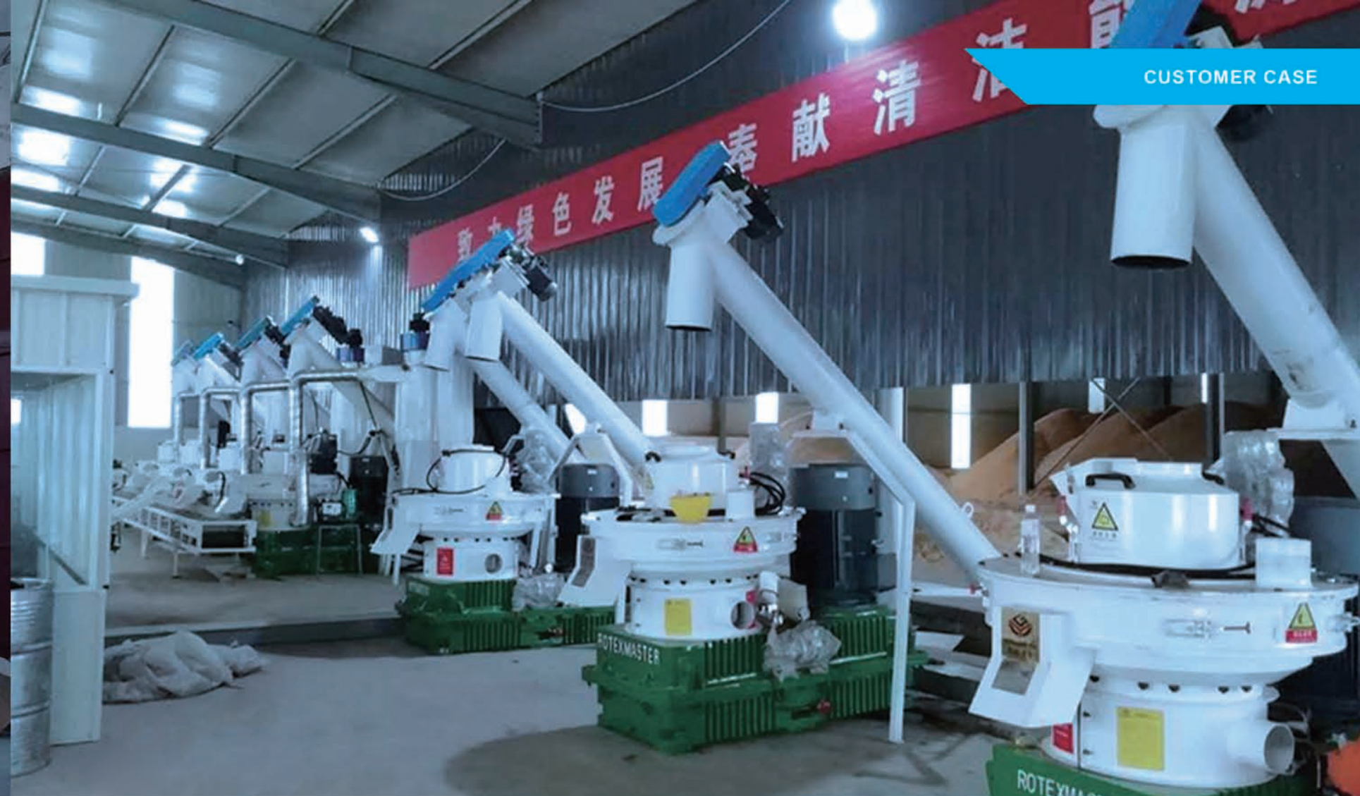
JIANGSU 10T/H WOOD PELLET PRODUCTION LINE
